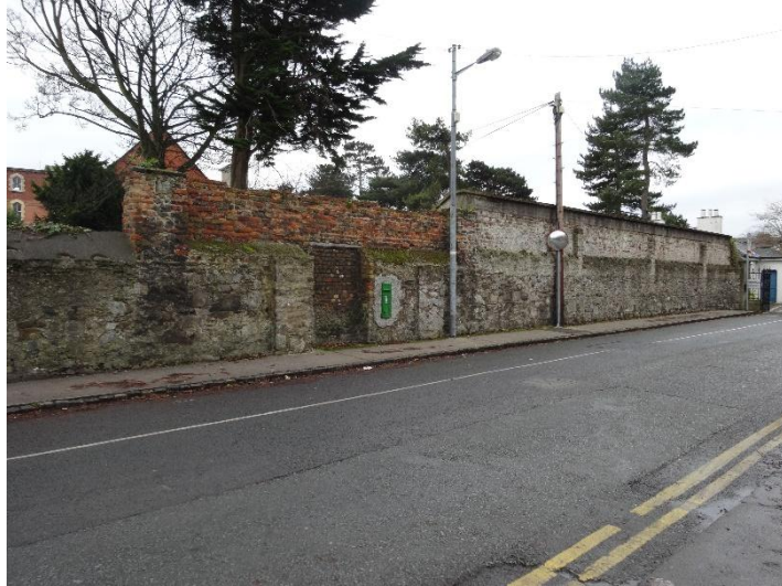
Rubble stone and brick northern boundary wall which forms boundary of site along Bloomfield Ave (Structure 11)
